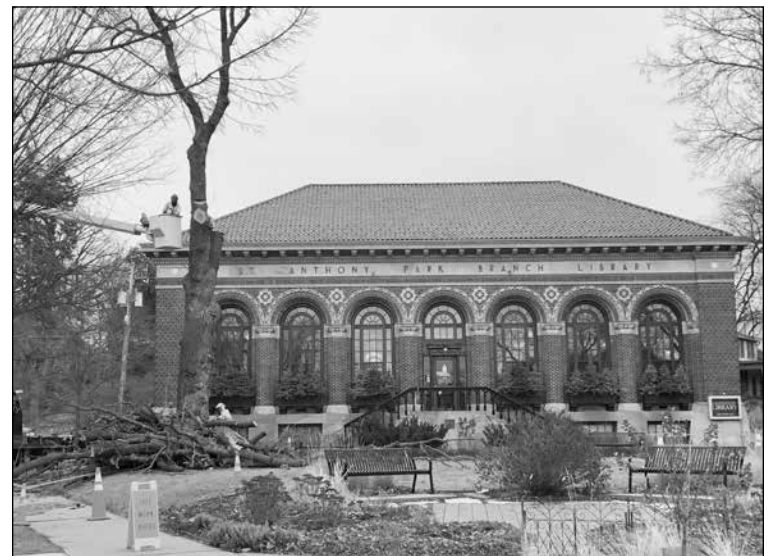
A work crew recently removed a dying giant white oak from the grounds of the St. Anthony Park Library. Photo by Rita La Doux.
